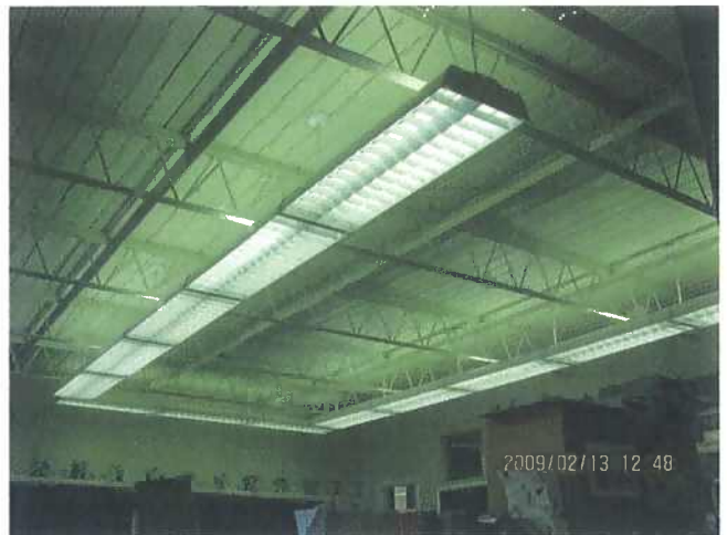
Electrical Picture #4 Typical Classroom Lighting
