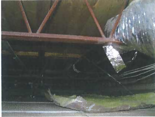
Mechanical Picture #7 ABS rain water leader with damaged insulation
