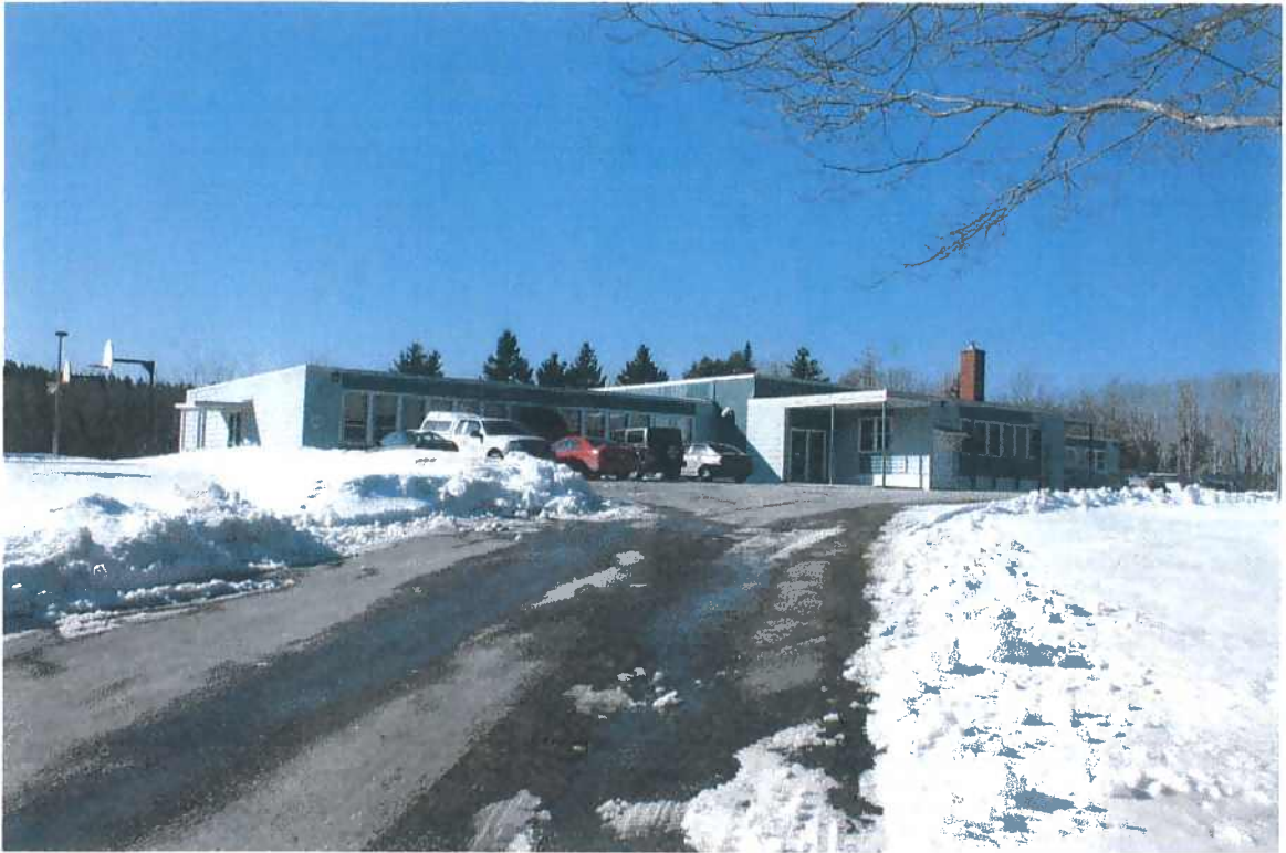
Figure 3 Pavement is in poor condition
