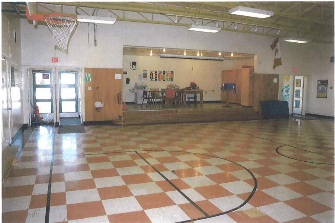
Figure 8 Gym / Multi purpose room. Note: lack of accessible access to stage. Principal's office and Administrative office are accessed from stage.
