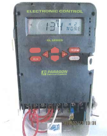
Electrical Picture #12 Class Dismissal Time Clock
