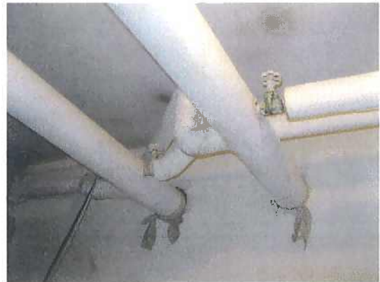
Mechanical Picture #6 Original gate valves (domestic water)
