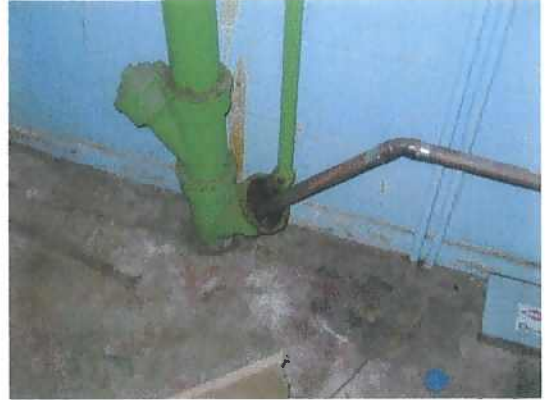
Mechanical Picture #8 Open cleanout on rainwater leader
