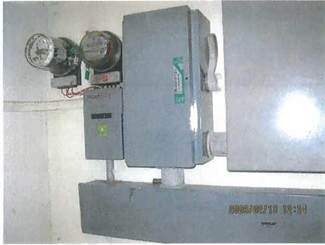
Electrical Picture #1 Electrical Service Entrance Equipment in Basement.
