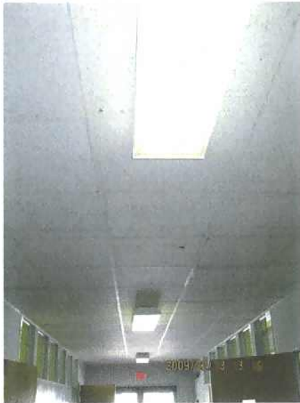
Electrical Picture #5 Typical Corridor Lighting
