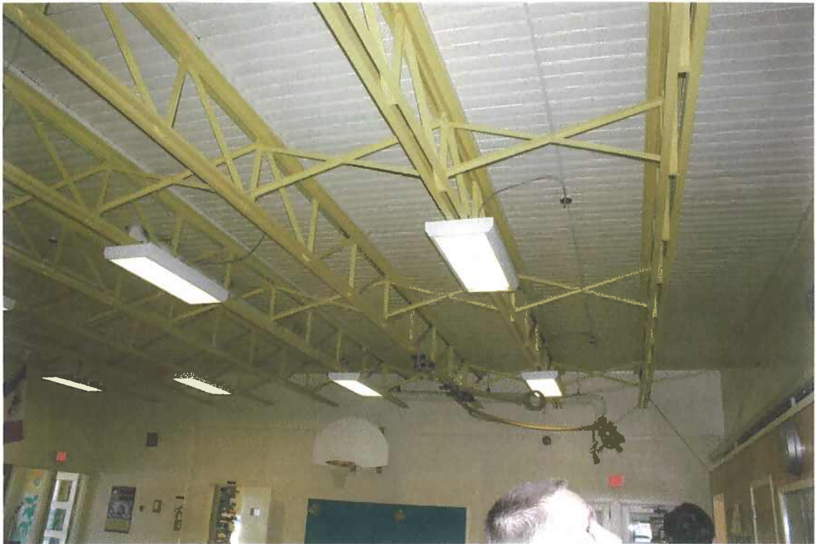
Figure 9 Exposed steel joints could be replaced with suspended acoustic tile ceiling to reduce noise.
