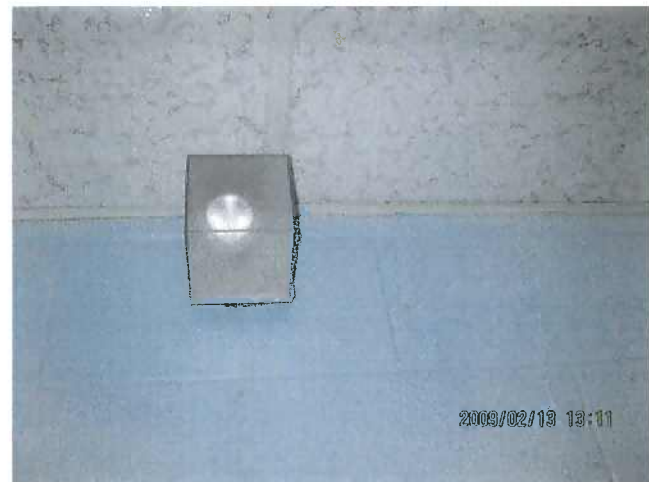
Electrical Picture #8 Typical Emergency Lighting Unit
