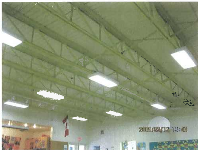
Electrical Picture #7 Multi Purpose Room Lighting
