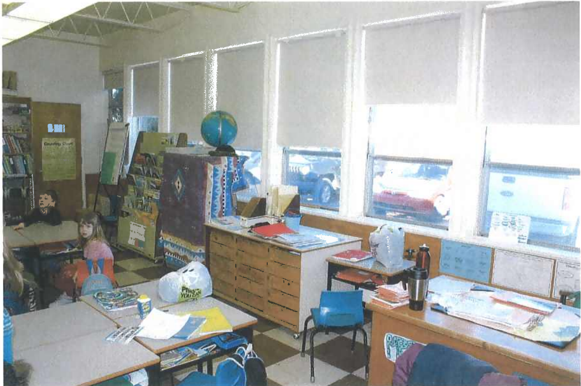
Figures 13 Windows and doors are 48 years old and need to be replaced.
