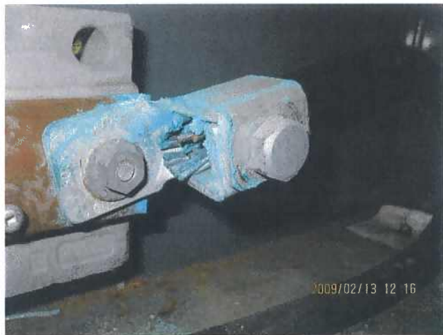
Electrical Picture #3 Electrical Basement Splitter Terminal Corrosion.
