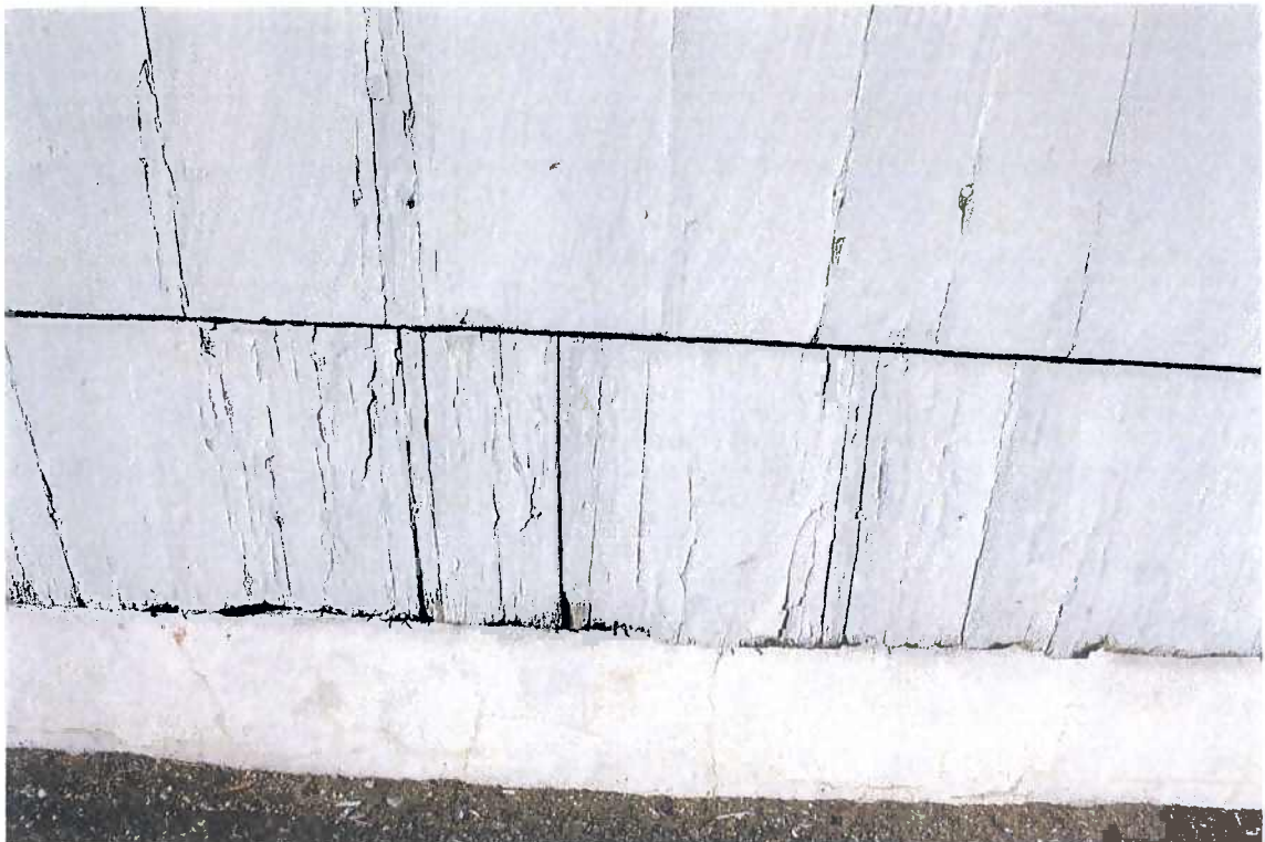
Figures 6 The lower courses of shingles should be replaced and the sheathing checked for rot. All remaining shingles should be scraped and painted.
