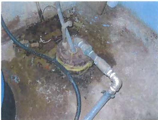
Mechanical Picture #5 Existing well in boiler room
