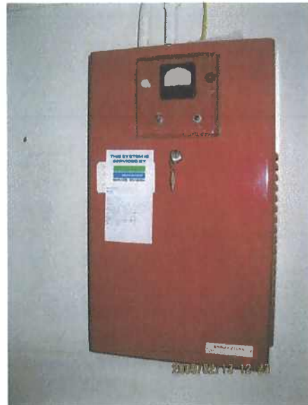
Electrical Picture #10 Fire Alarm Panel
