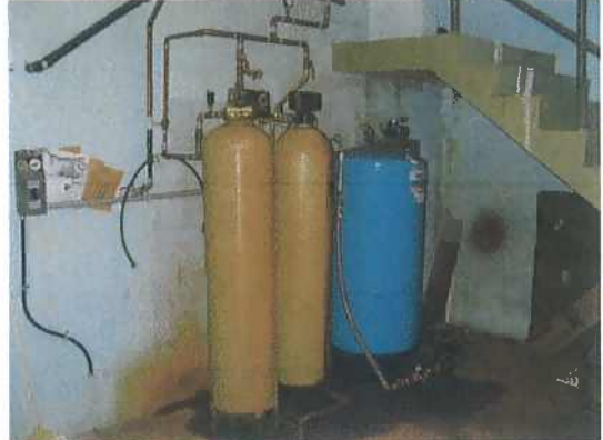
Mechanical Picture #4 Water system
